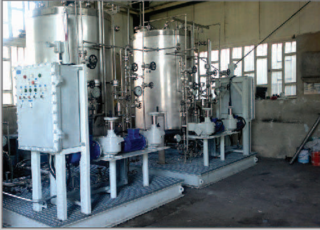
Corrosion Inhibitor Package
