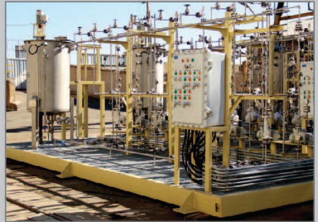
Corrosion Inhibitor Package
