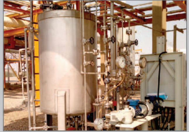
Chemical Injection Package
